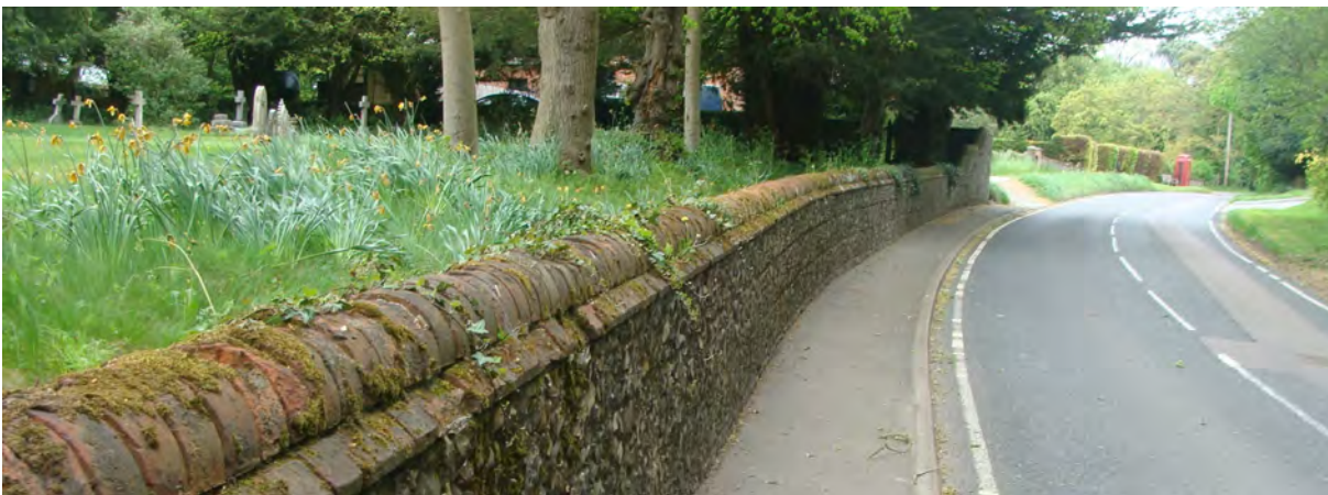
Picture 1.14 The wall surrounding the churchyard is an important and strong feature in the street scene
